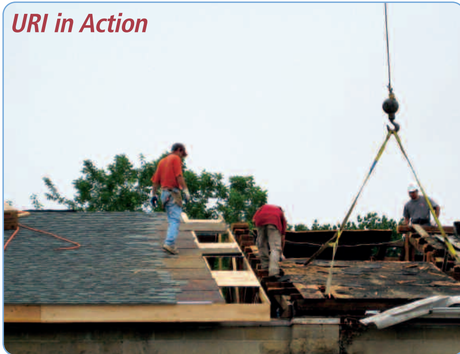
URI personnel working on removal and re-construction of a fire damaged roof in Maryland.
